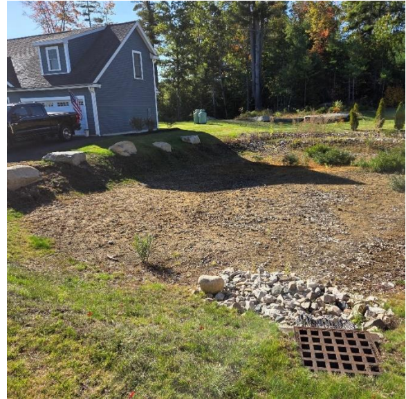
ADD'L RIP-RAP REQ'D DUE TO RUNOFF FROM PARKING AREA
